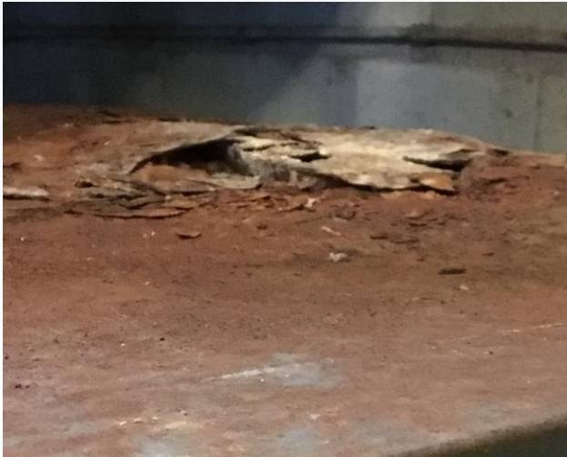
Corrosion on Boiler
