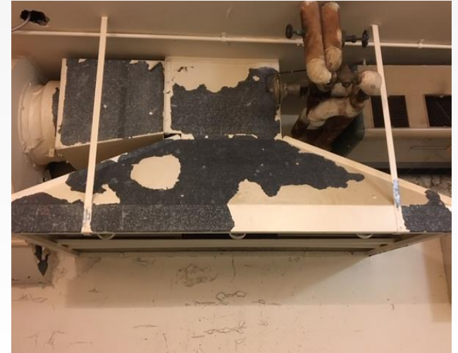
Deteriorated System in Kitchen
