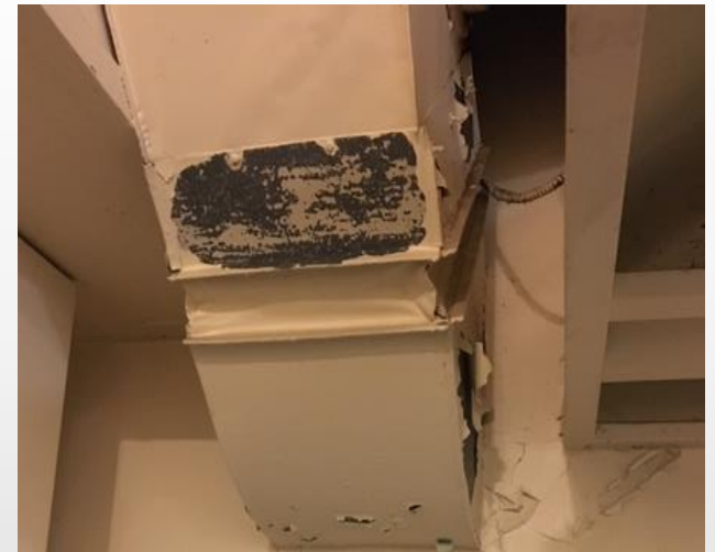
Peeling Paint in Kitchen
