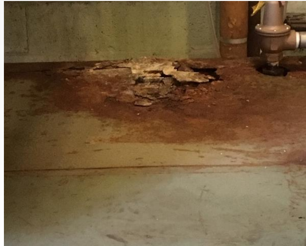
Corrosion on Boiler
